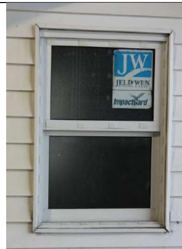
Figure 10: Windows showing location of 3M® Dual Lock® Reclosable Fasteners.
